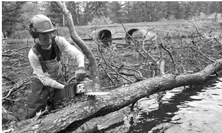
Important habitat restoration work like this, on the Au Sable River, is supported by funding from the Aquatic Habitat Grant Program, administered by the Michigan DNR. In 2018, $1.25 million in funding is available to local, federal, state and tribal governments and nonprofit groups. (photo by David Kenyon of DNR)
